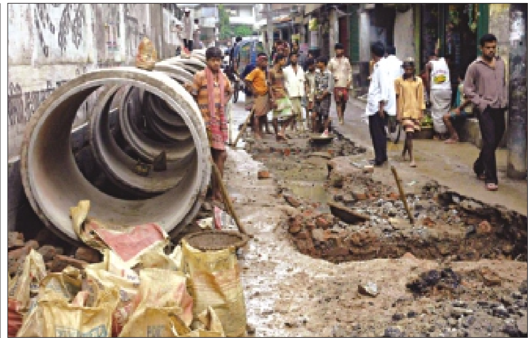
The slow pace of work on installing sewerage pipes causes sufferings to the residents of Tally Office Road at Rayerbazar in the capital.
