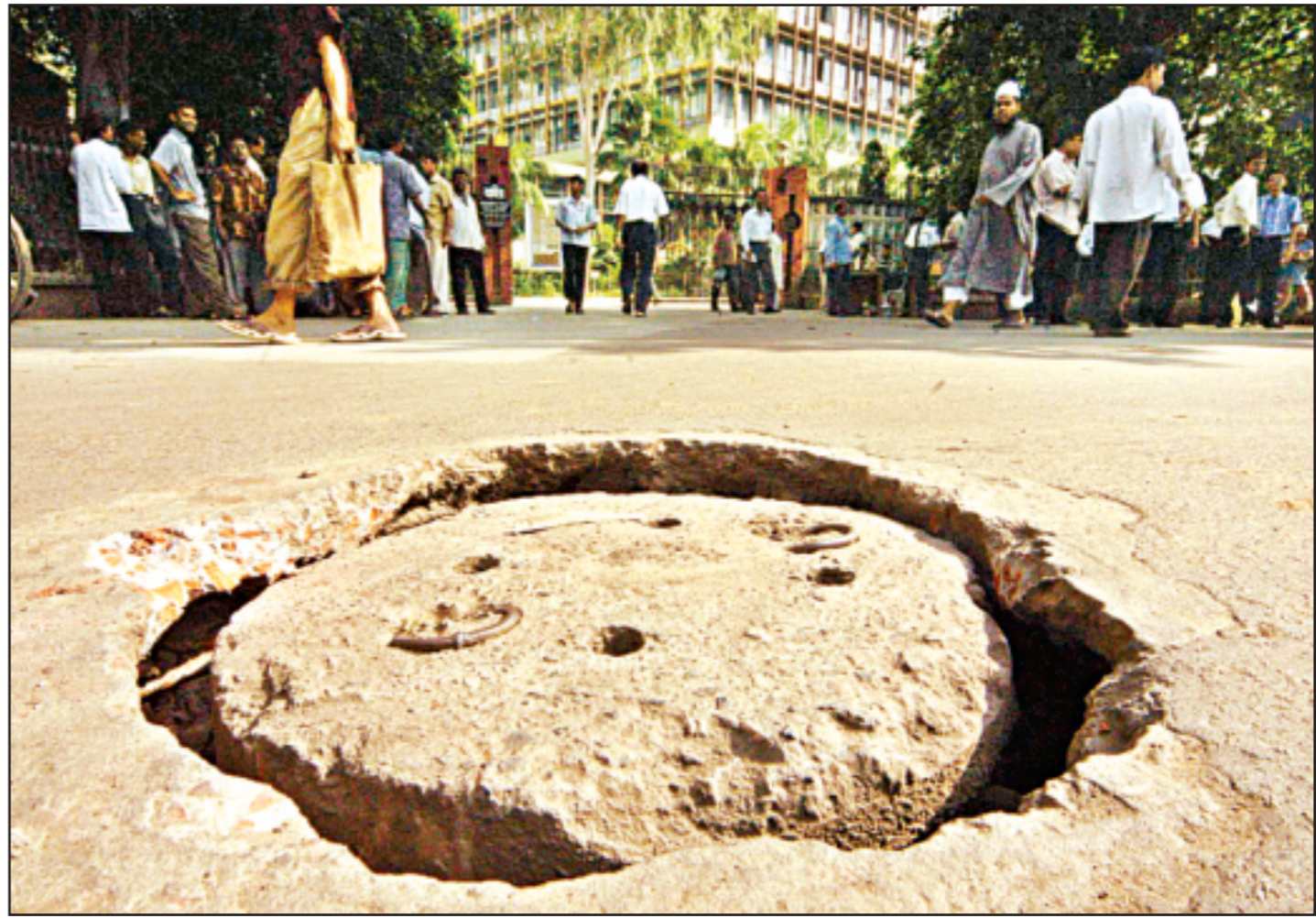
PHOTO: STAR A run-down manhole on Motijheel-Kamalapur link road near the second gate of Bangladesh Bank poses danger to pedestrians as well as passengers.
