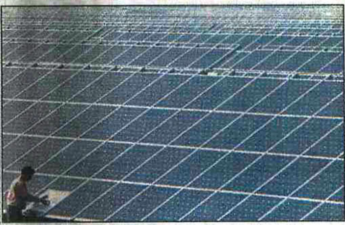
Project leader Martin Bucher is working on a solar power module in Pocking in Lower Bavaria.
