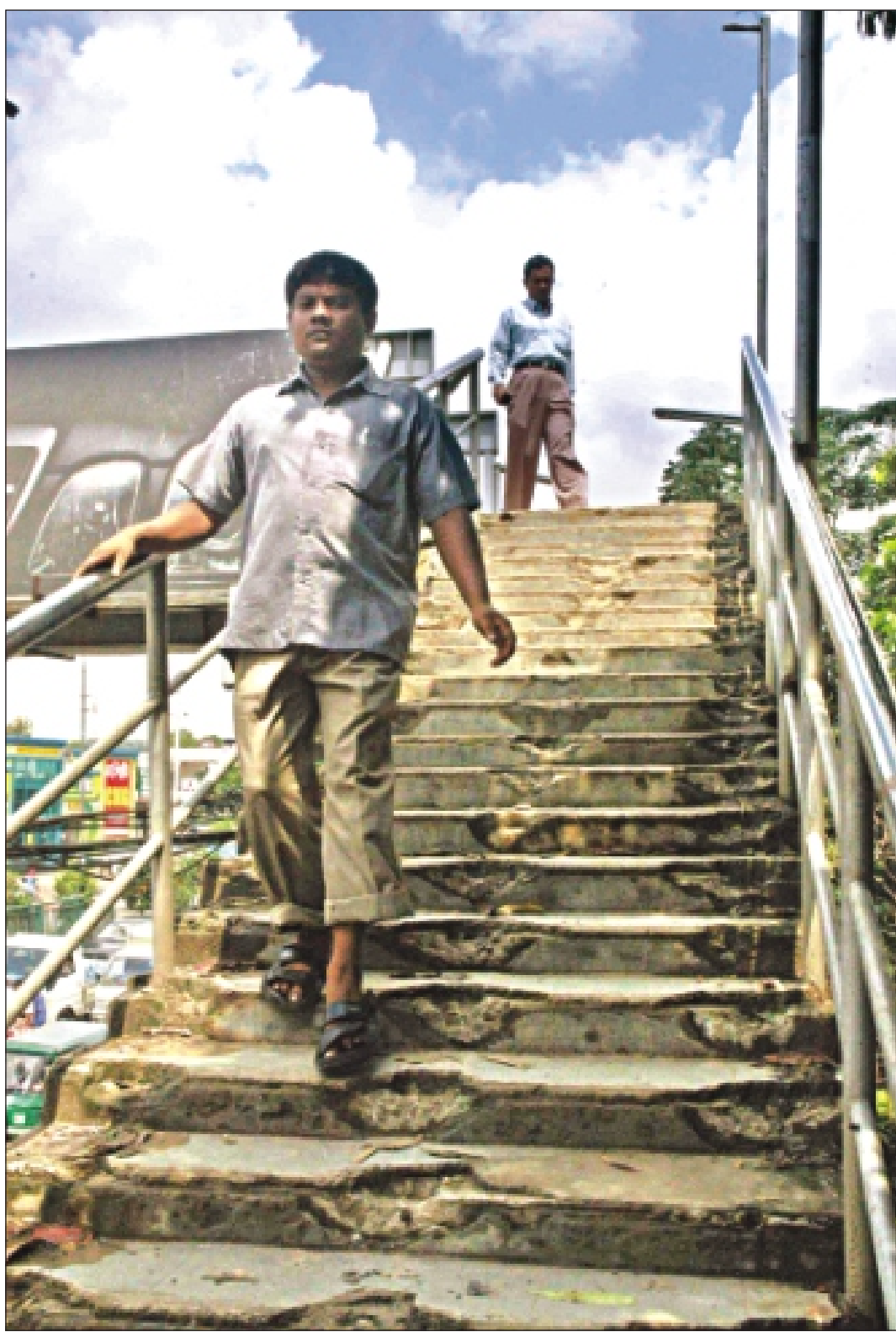
A man climbs down the worn out stairs of a foot over-bridge in front of the Dhaka Polytechnic Institute at Tejgaon in the capital yesterday as the authorities concerned turn a blind eye to the bridge's repair needs.
