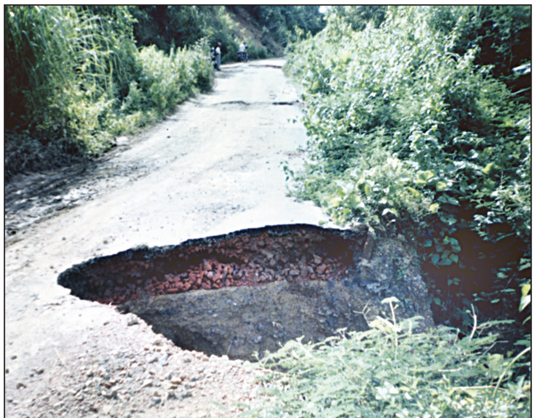
The Khagrachhari-Baghaichhari road has become a death trap as it collapsed at many points due to rain. The photo was taken from Marisshah. Officials said the road can not be repaired due to lack of funds.
