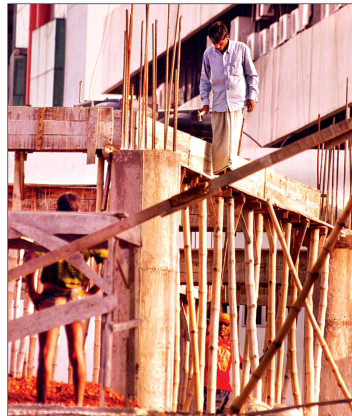
Construction workers on an under-construction building without any safety gear.
