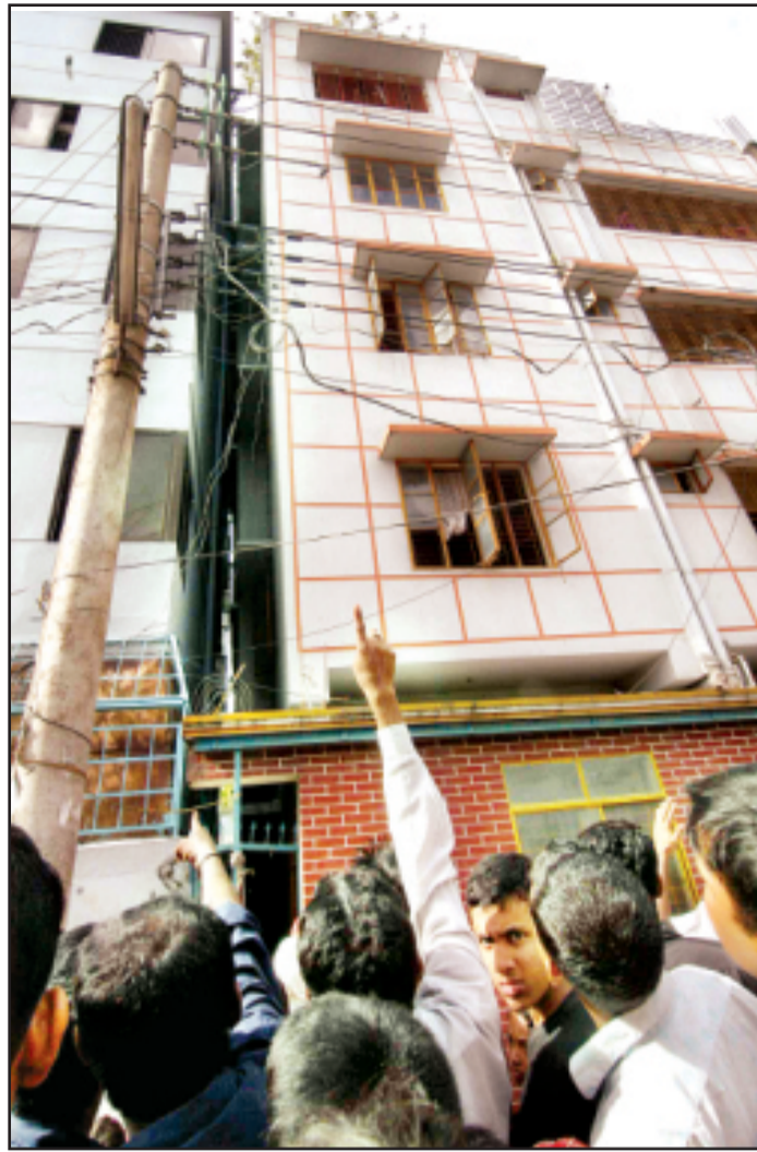
PHOTO: STAR Hundreds of people thronged to Road -17 in Rupnagar Residential Area of Mirpur in the city yesterday to see the two adjoining buildings tilted towards each other.
