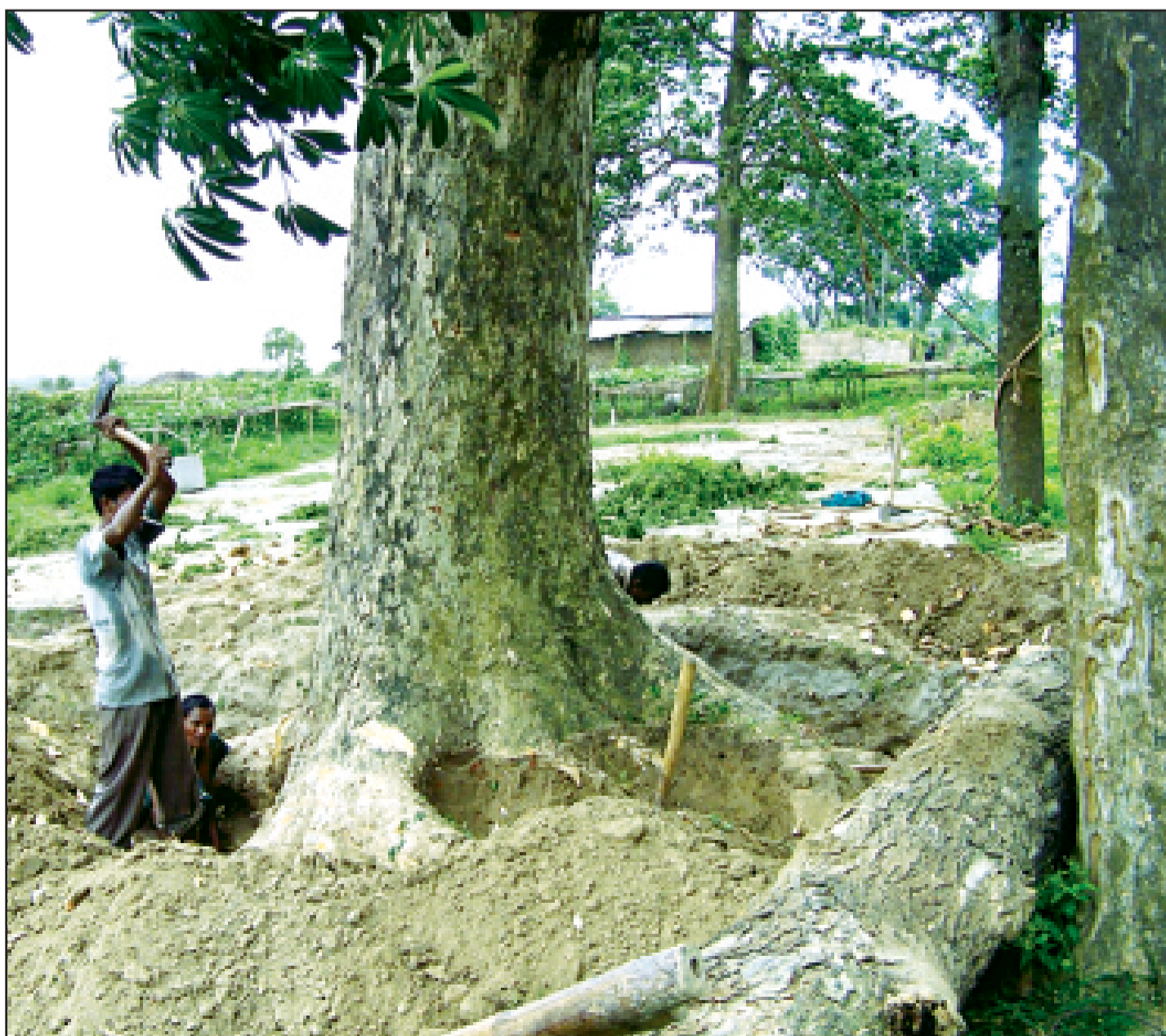
A worker cuts down an ancient tree in Rajshahi Town Protection Embankment area yesterday. An influential person is behind the felling of a number of trees, an act that poses a threat to the embankment.
