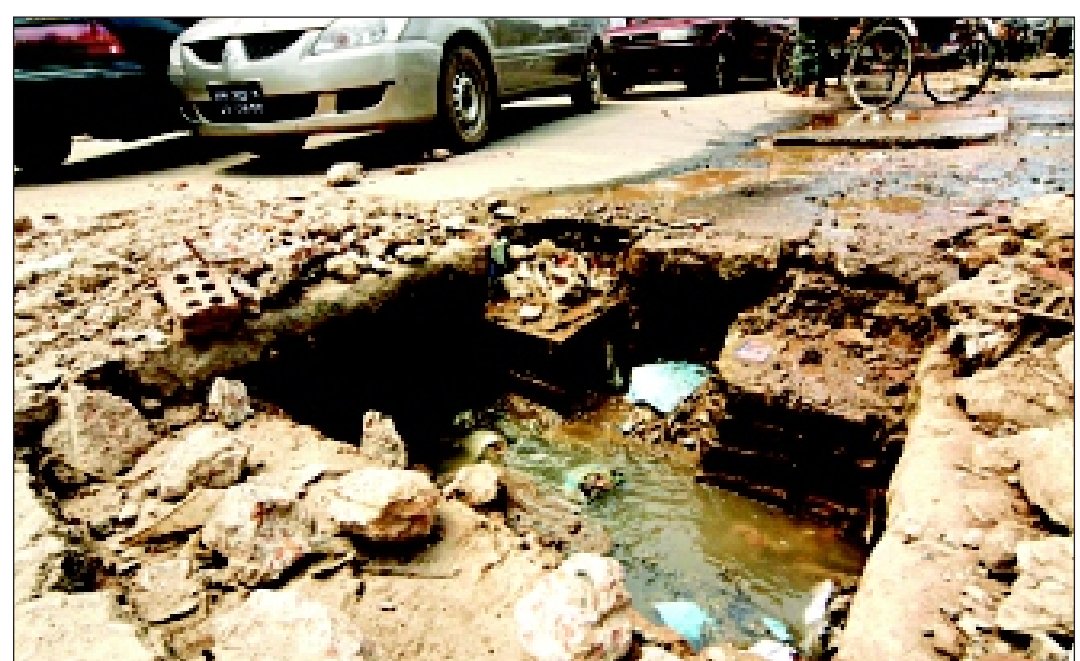
Opening of this sewer near Gulshan-1 intersection is missing its concrete lid. The gaping hole not only spreads odour but also poses threat to pedestrians and vehicles plying the street.
