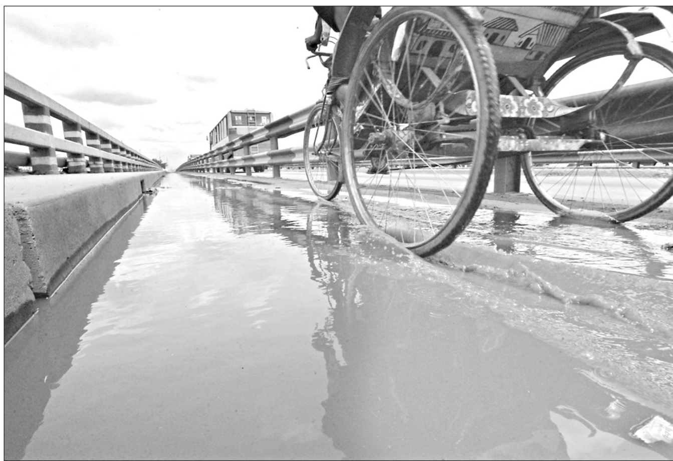
A waterlogged Aminbazar bridge at Gabtoli is a common sight whenever it rains.
