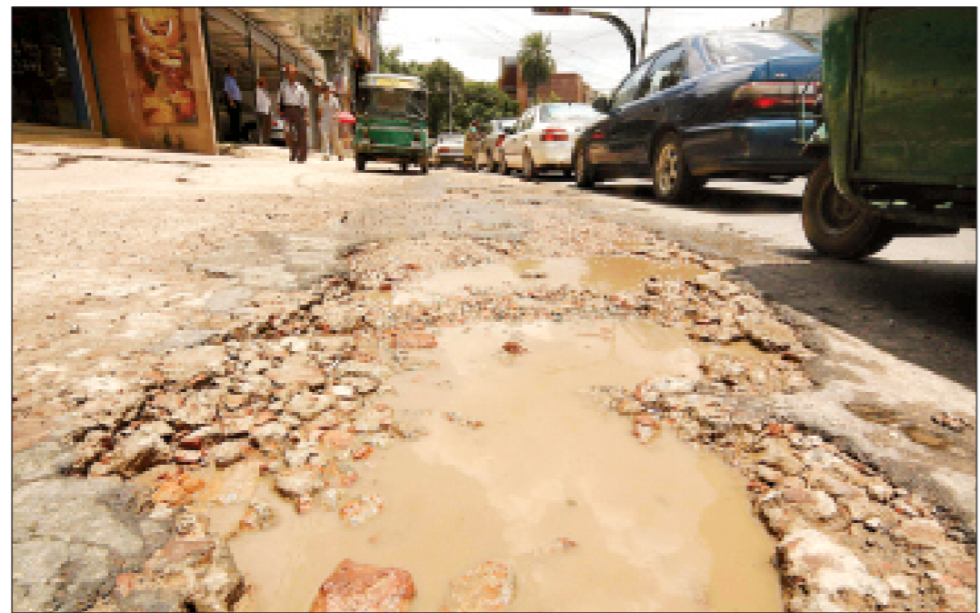
Residents of Dhanmondi and users of Road-27 continue to suffer as the authorities concerned after digging into the road just filled it up with dirt without paving it.
