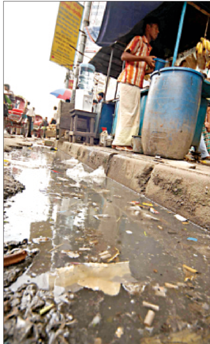
Drain water stagnates in the broken part of a road adjoining the Purana Paltan intersection in the capital.
