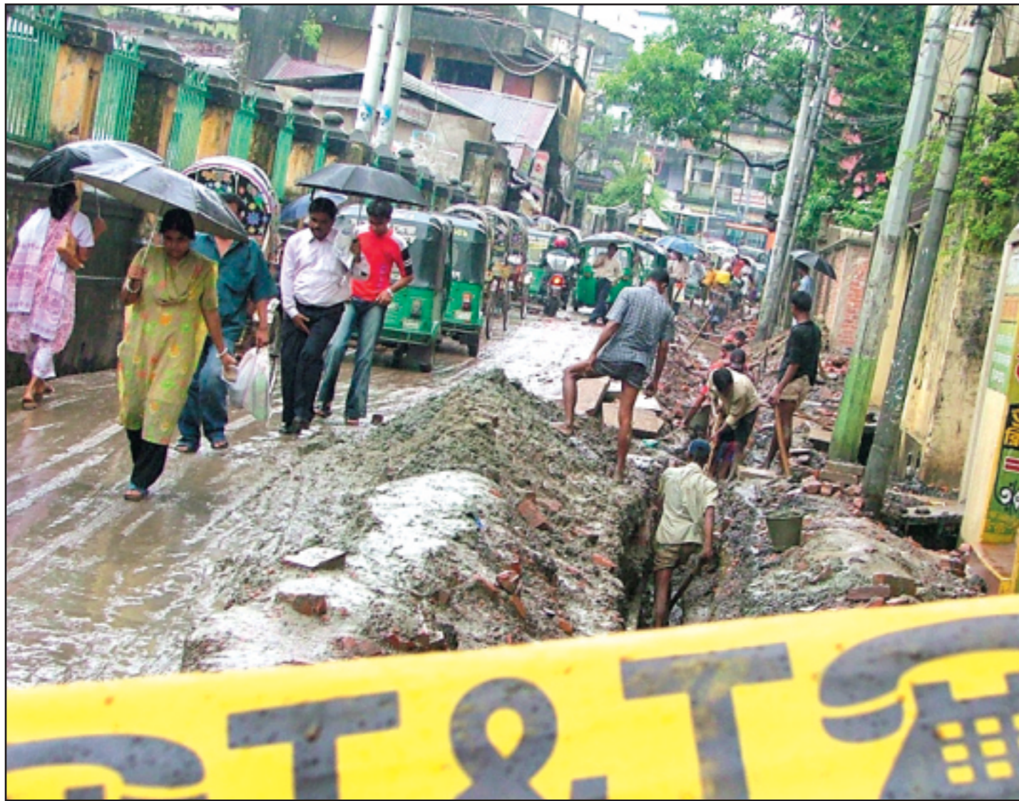
Road digging by the BTTB during the monsoon season has added to the suffering of the passers-by in Chittagong city. This picture was taken from Rahmatganj area yesterday. PHOTO: STAR
