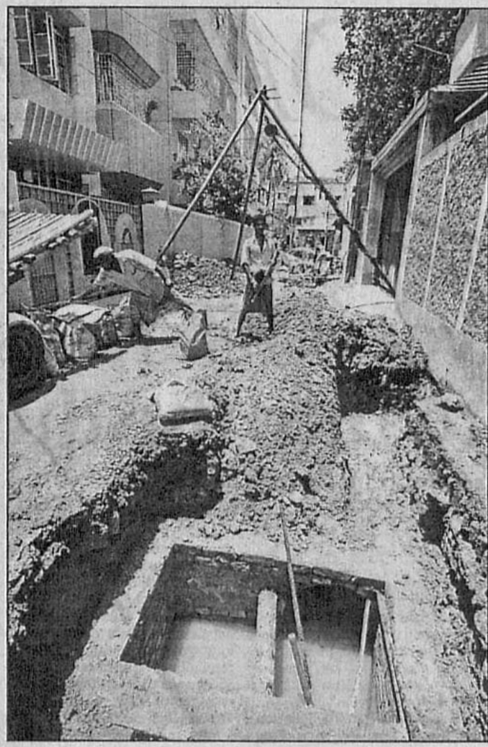
Work on laying of sewer pipes has been going on at a road at Ahmabagh in the city for over a week, causing suffering to passers-by.
