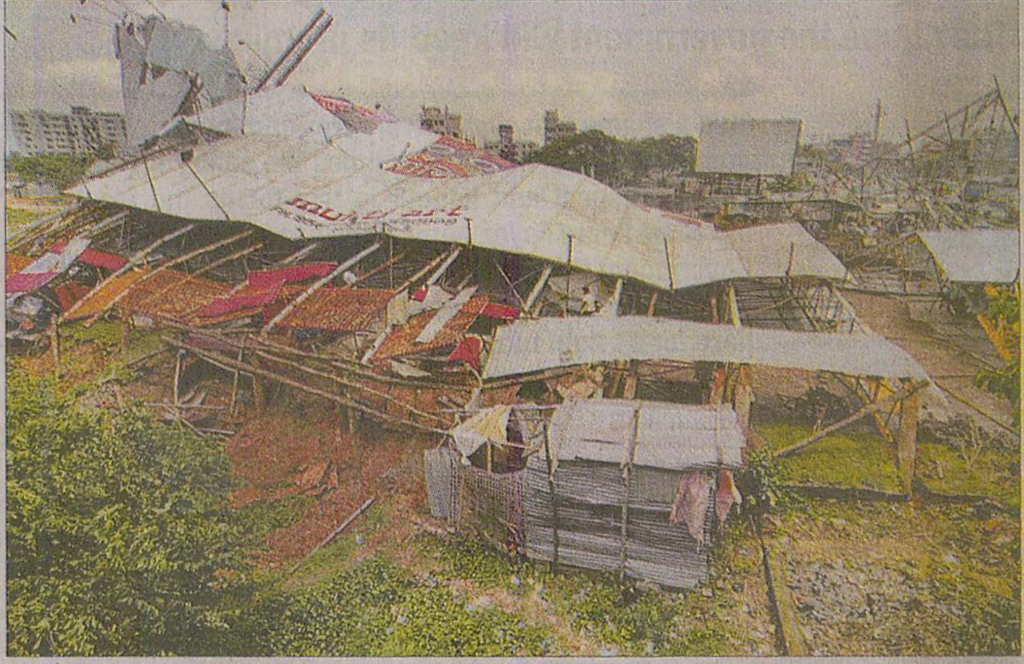
Billboards that collapsed on a filling station on Pragati Sarani during a storm on June 16 and killed two people have not been removed yet.
