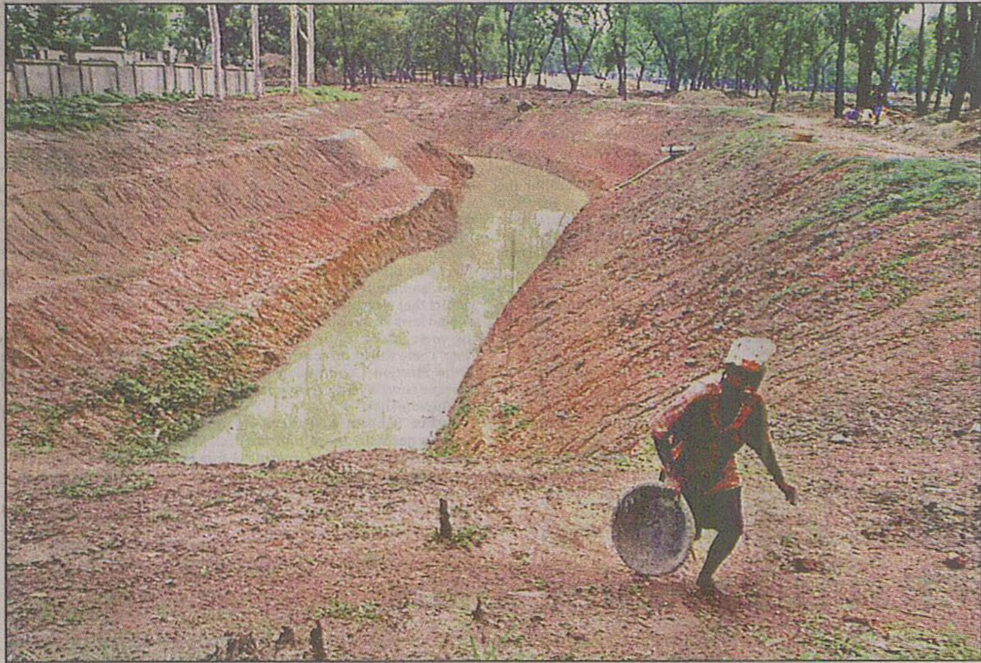
Dhaka City Corporation has been digging a lake at the Osmani Udyan in the city after felling many trees.
