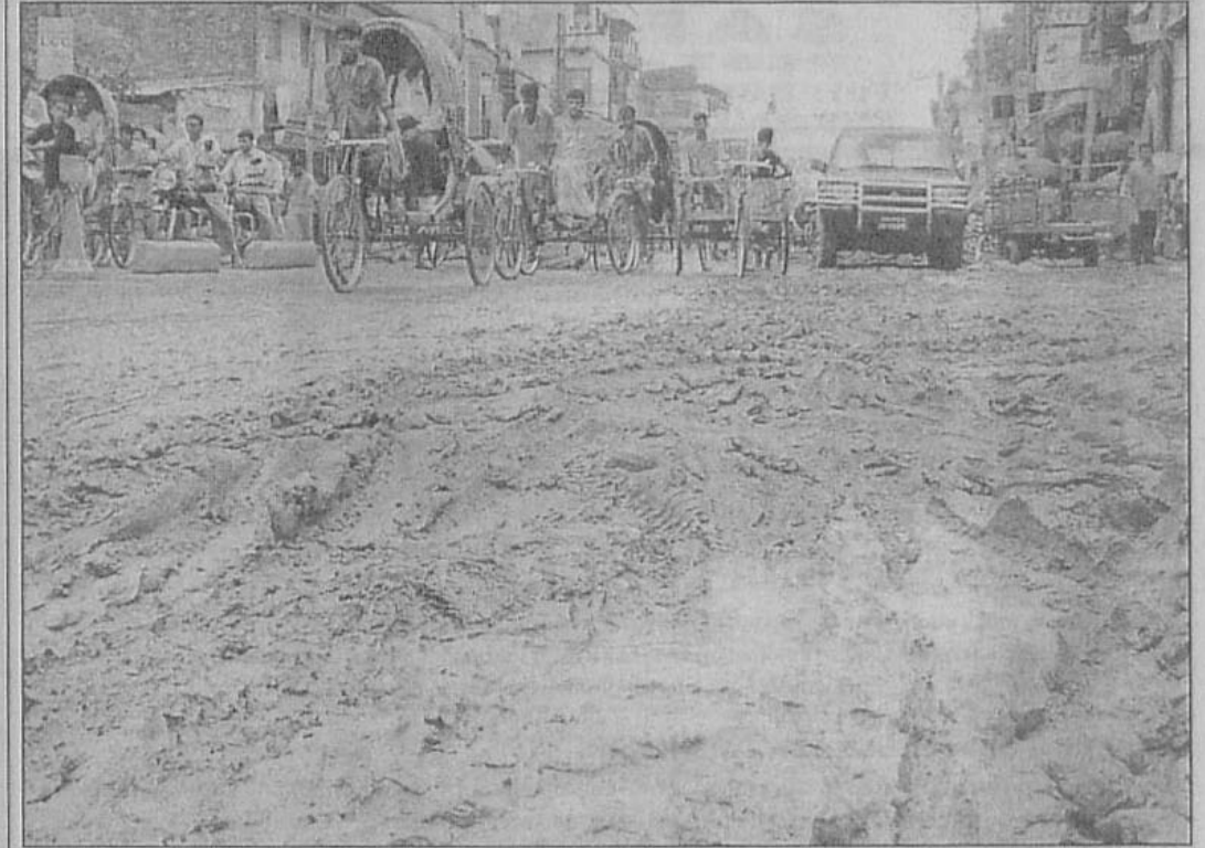
Accumulated mud on the under construction Kabi Nazul Islam Sarak hinders smooth plying of vehicles and movement of passers-by in Bogra. The road construction has been stalled due to alleged negligence of contractors and fund constraint.
