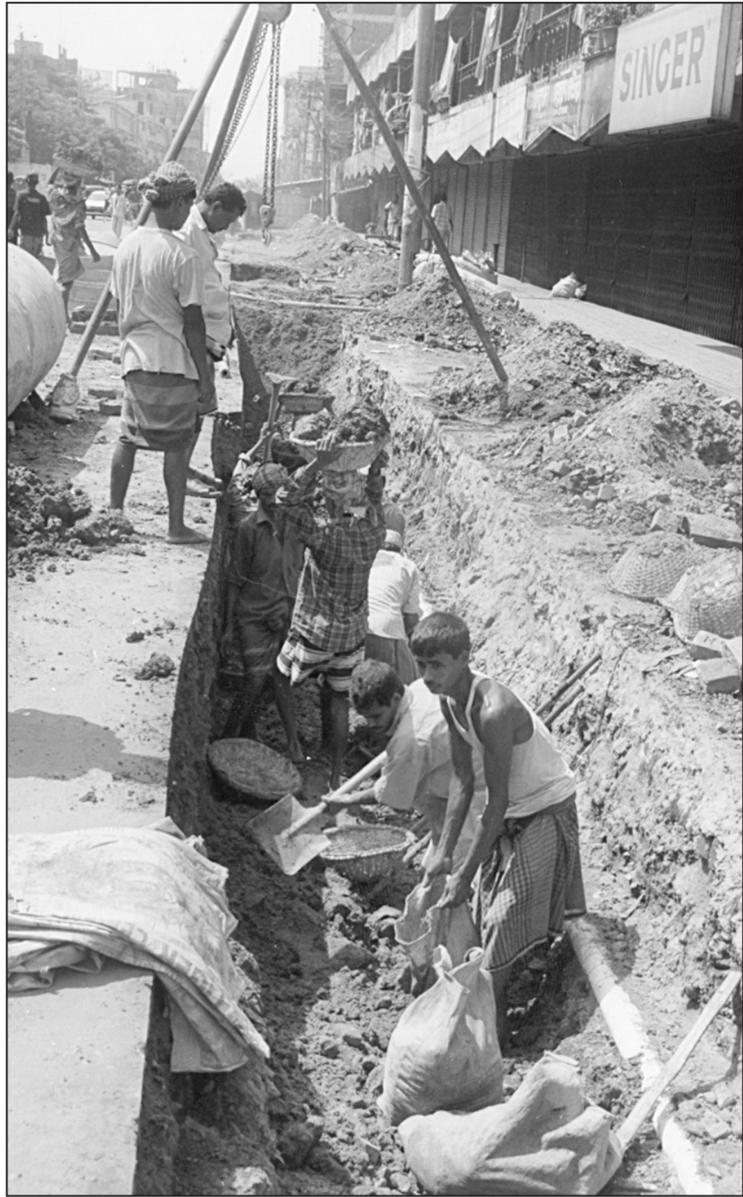
Road digging at Swamibagh in the city has been going on for about a month, causing inconvenience to the commuters. Situation will get worse as monsoon looms.
