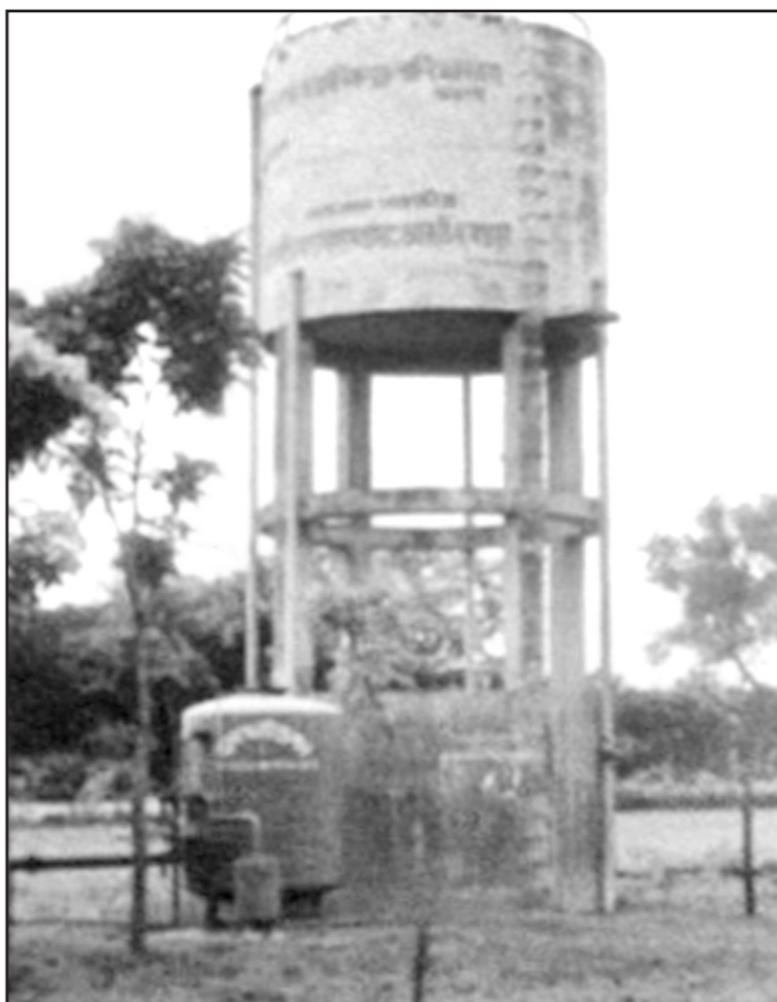
PHOTO: STAR The overhead tank and water treatment facilities lying ideal for about 11 months in Kalaroa.
