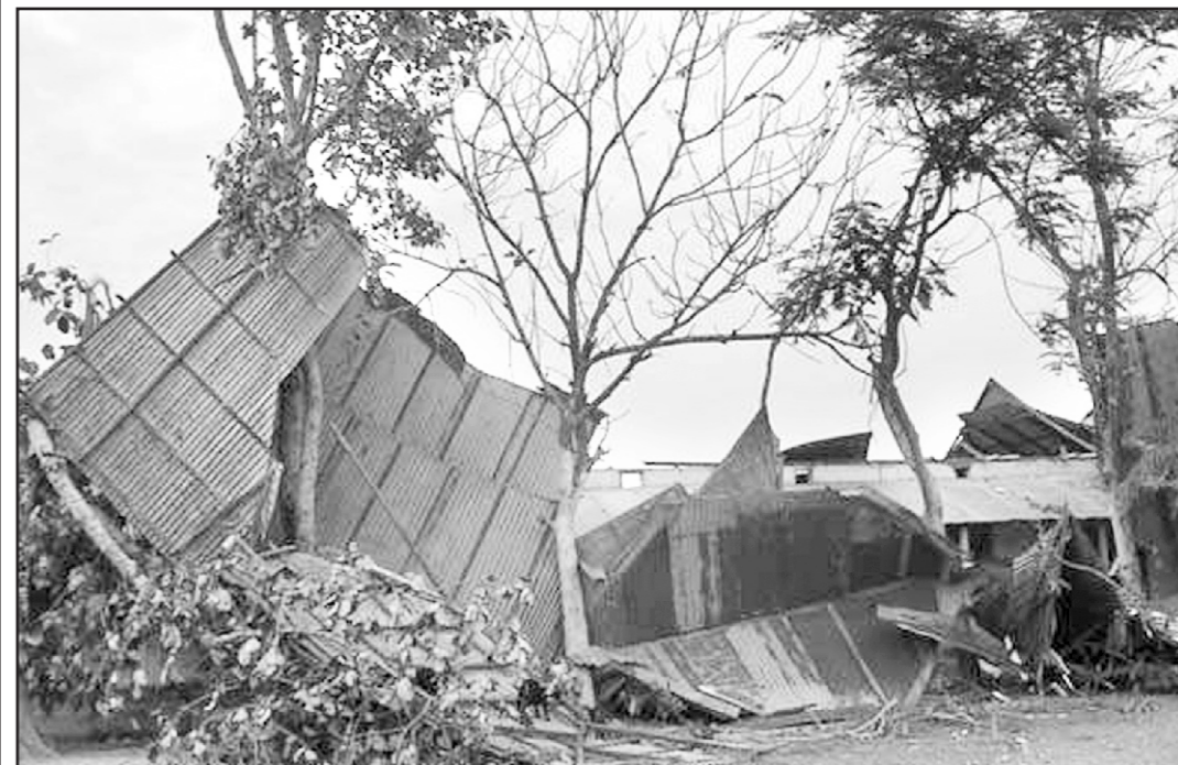
PHOTO: STAR The Gonda High School in Kendua, one of the many structures tore down by Sunday's nor'wester in Netrakona.
