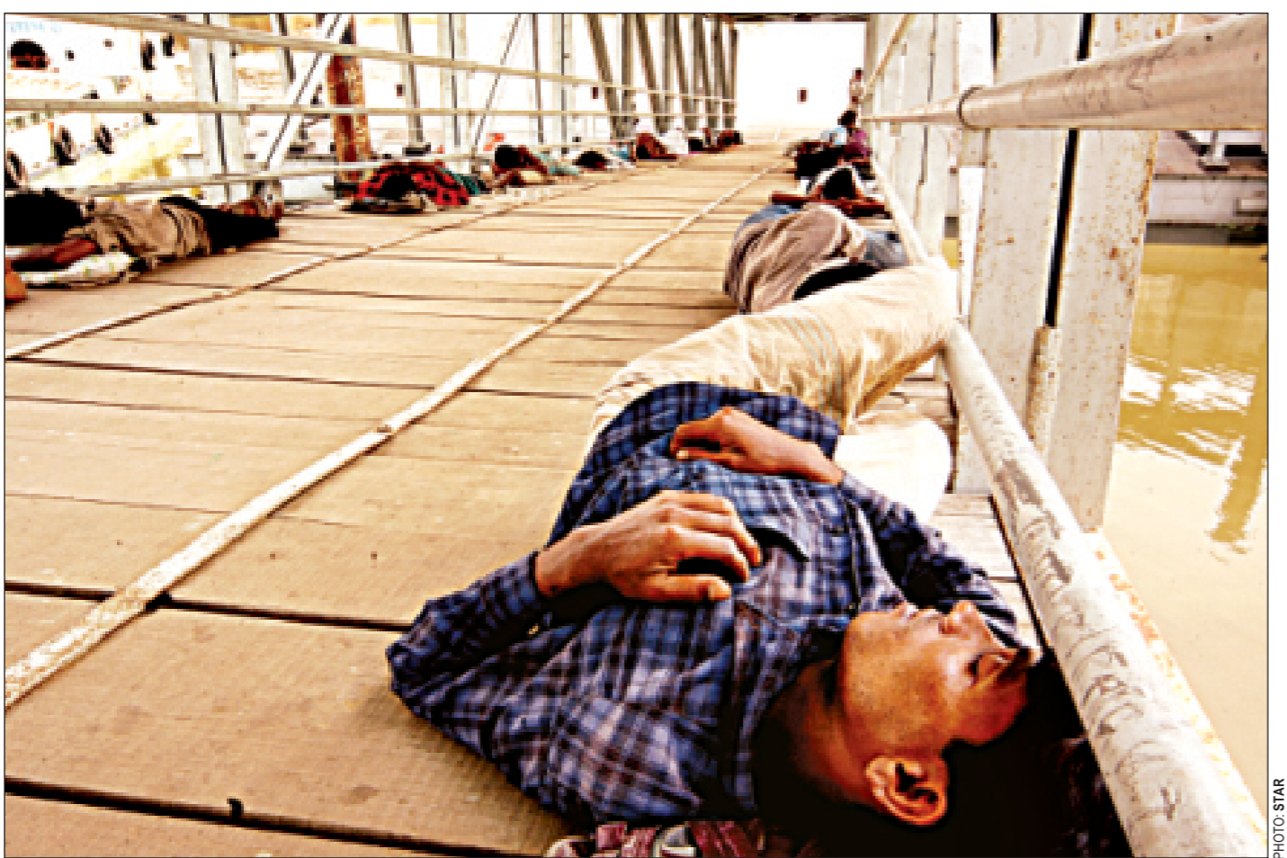
The gangway to a jetty for passenger launches on the much-publicised city circular waterway near the bridge at Amin Bazar is lying unused. Floating people now sleep on the gangway as the waterway inaugurated amid fanfare was partly operational only for a few weeks.
