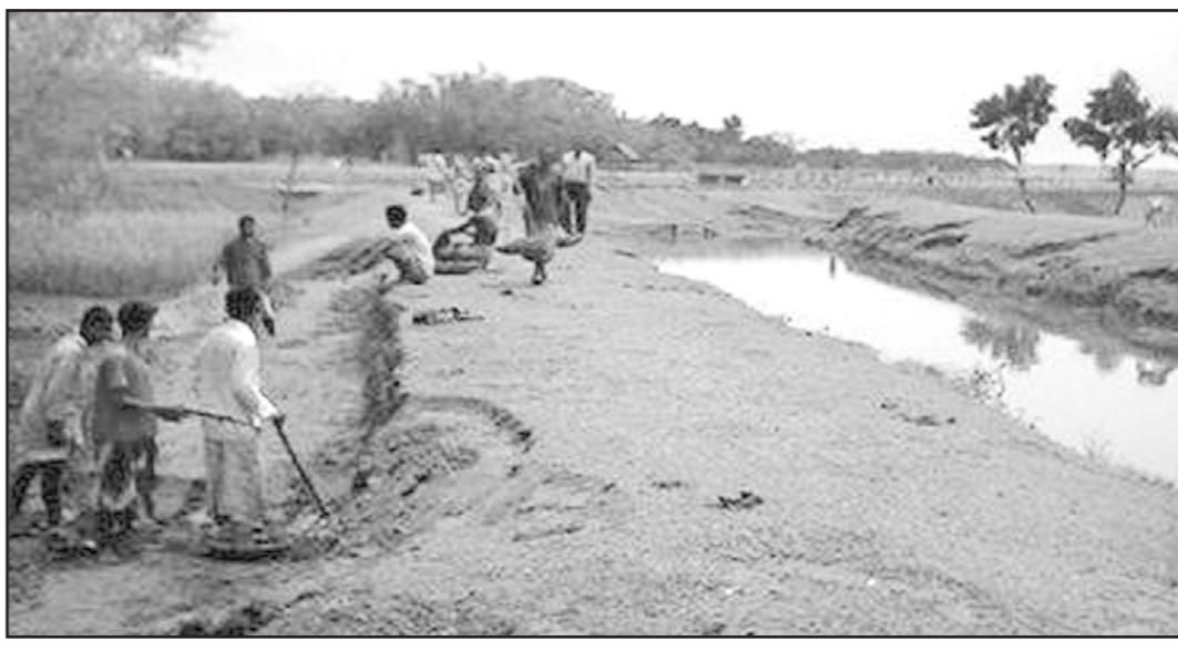
PHOTO: STAR Labourers cutting earth from the bank of a branch canal of Teesta Irrigation Project (TIP) in Jaldhaka to repair an embankment.
