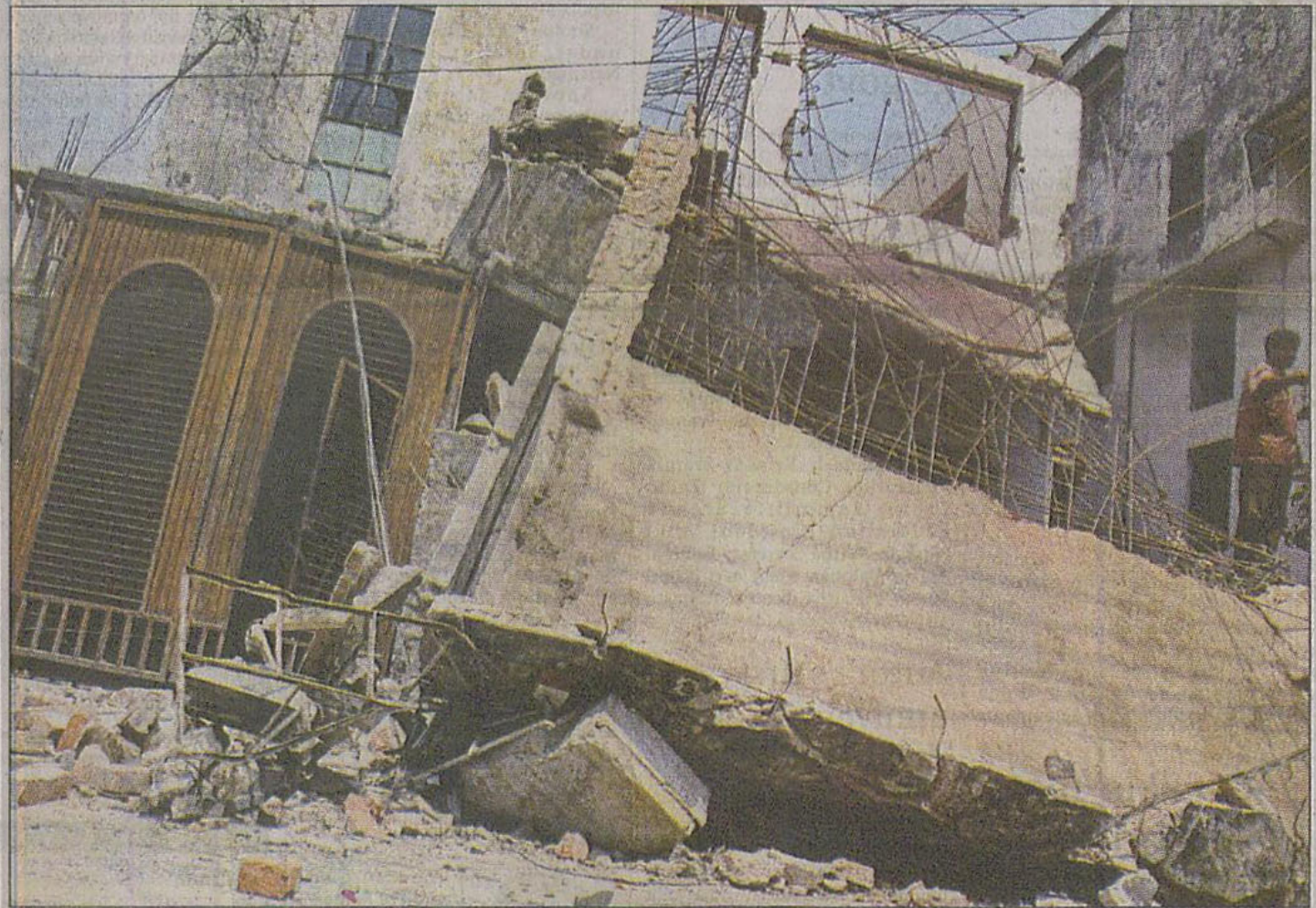
This chunk of the roof of a two-storey building in Tajmahal Road of Mohammadpur in the city fell on a car parked in front yesterday during its demolition to make room for a new apartment complex. Luckily, no one was hurt in the incident.
