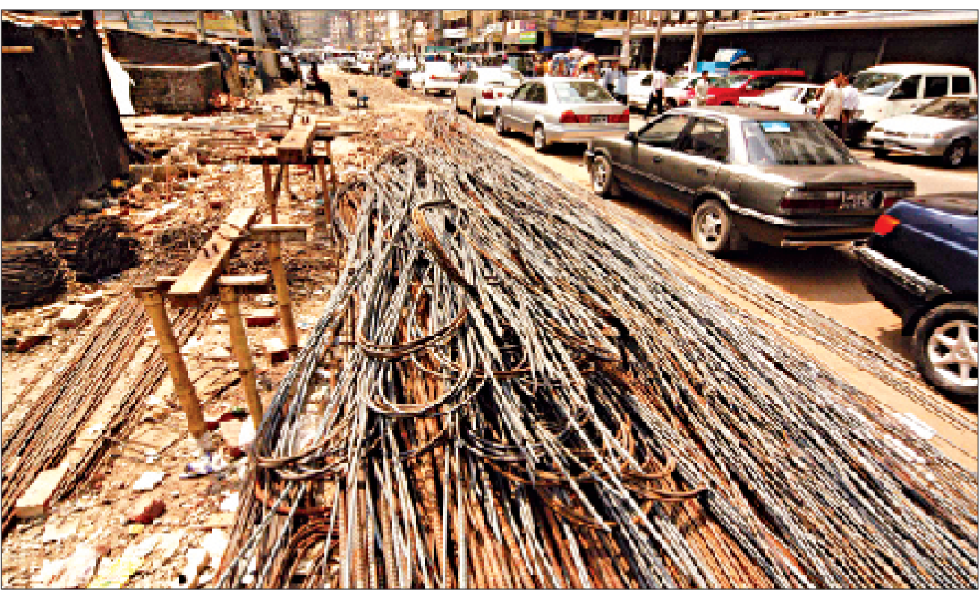
Iron rods for construction are piled up occupying almost half of a busy street in Dilkhusha in the capital.
