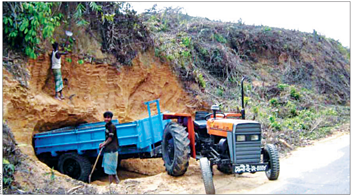
Despite an official ban, illegal hill cutting continues unabated in Khagrachhari.
