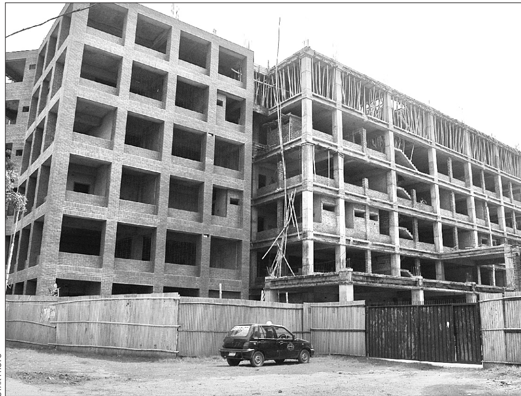
An under construction extended part of Dhaka Dental College and Hospital in Mirpur.
