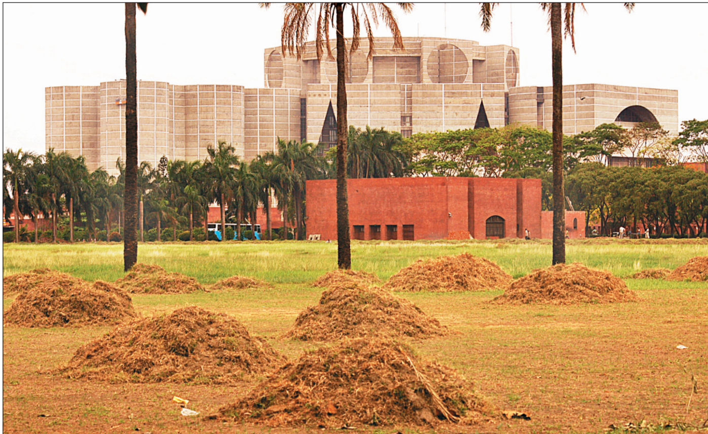
Mounds of earth stacked at certain points on the Sangsad Bhaban lawn as a result of its development work.
