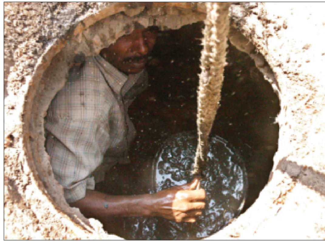
Despite five deaths in the last three months while cleaning manholes in the capital, two cleaners yesterday work in Kamalapur without any safety measures.
