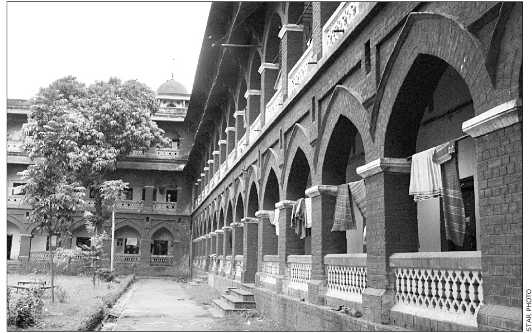
North block of FH Hall is the most vulnerable putting lives of students at grave risk.
