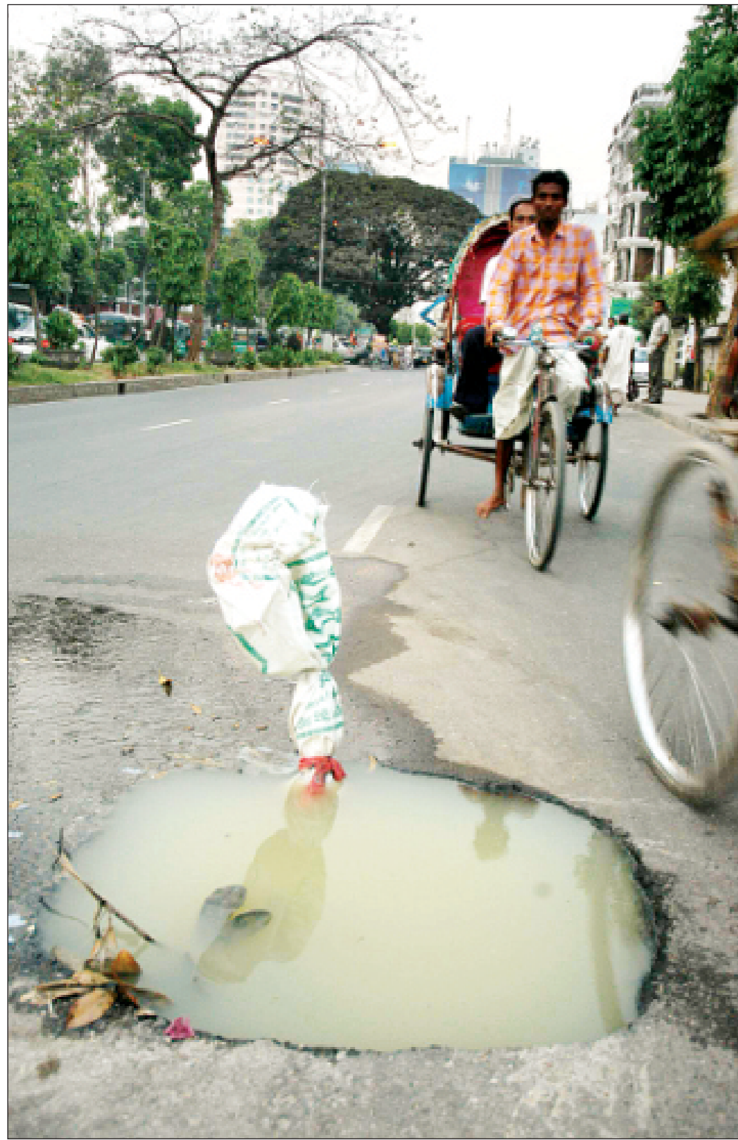
A polythene bag tied to a stick is the only sign that warns of an open manhole on a road near Gulshan-1 in the city. The lid was stolen months ago and the manhole now spreads unbearable stench. Besides, sewerage water floods the road with passing vehicles spraying the filth.
