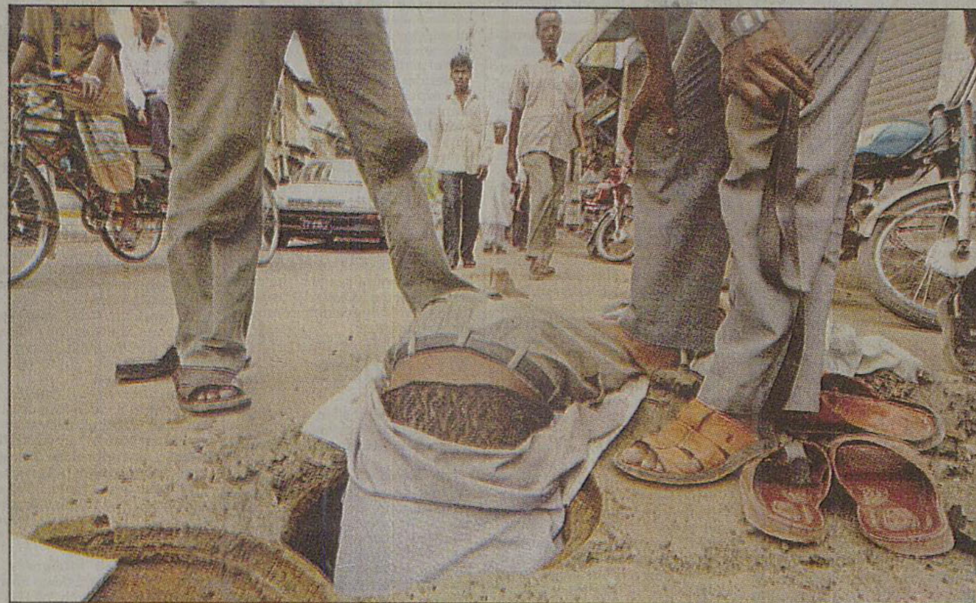
LURKING DANGER... A plumber dangles half his body through a manhole to repair a leak in the water supply line on Motijheel-Kamalapur Road yesterday while co-workers hold him with their feet on his knees.
