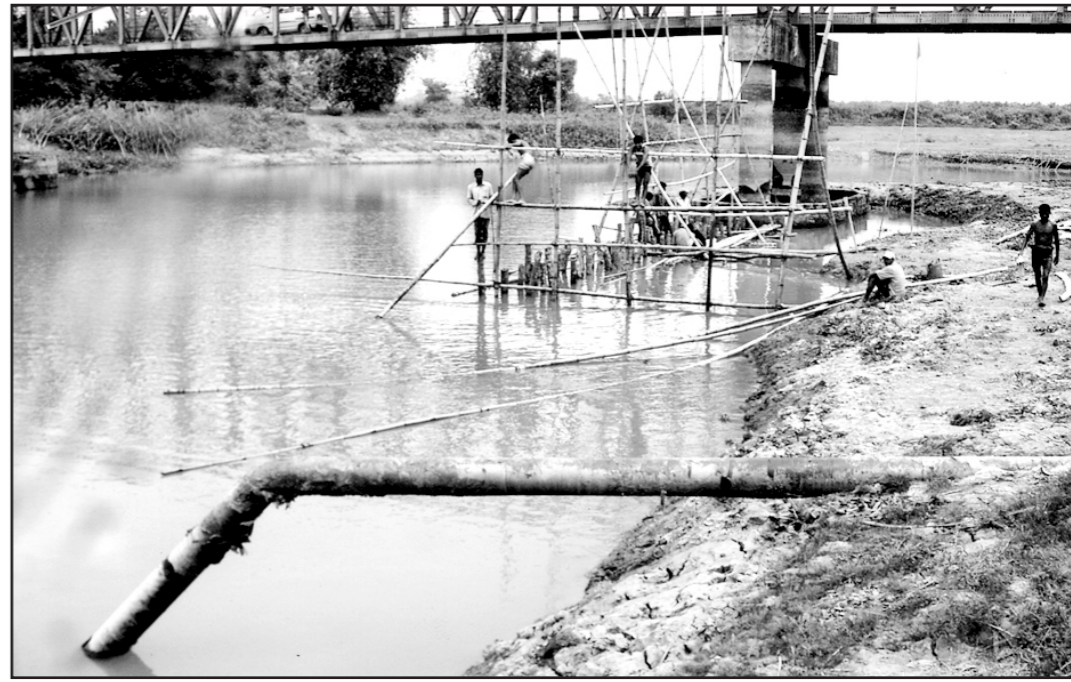
Unprotected gas pipeline ... The pipeline supplying gas from Jalalabad gas field to Fenchuganj Fertiliser Factory has surfaced near Sylhet city as erosion has removed soil, making it vulnerable.
