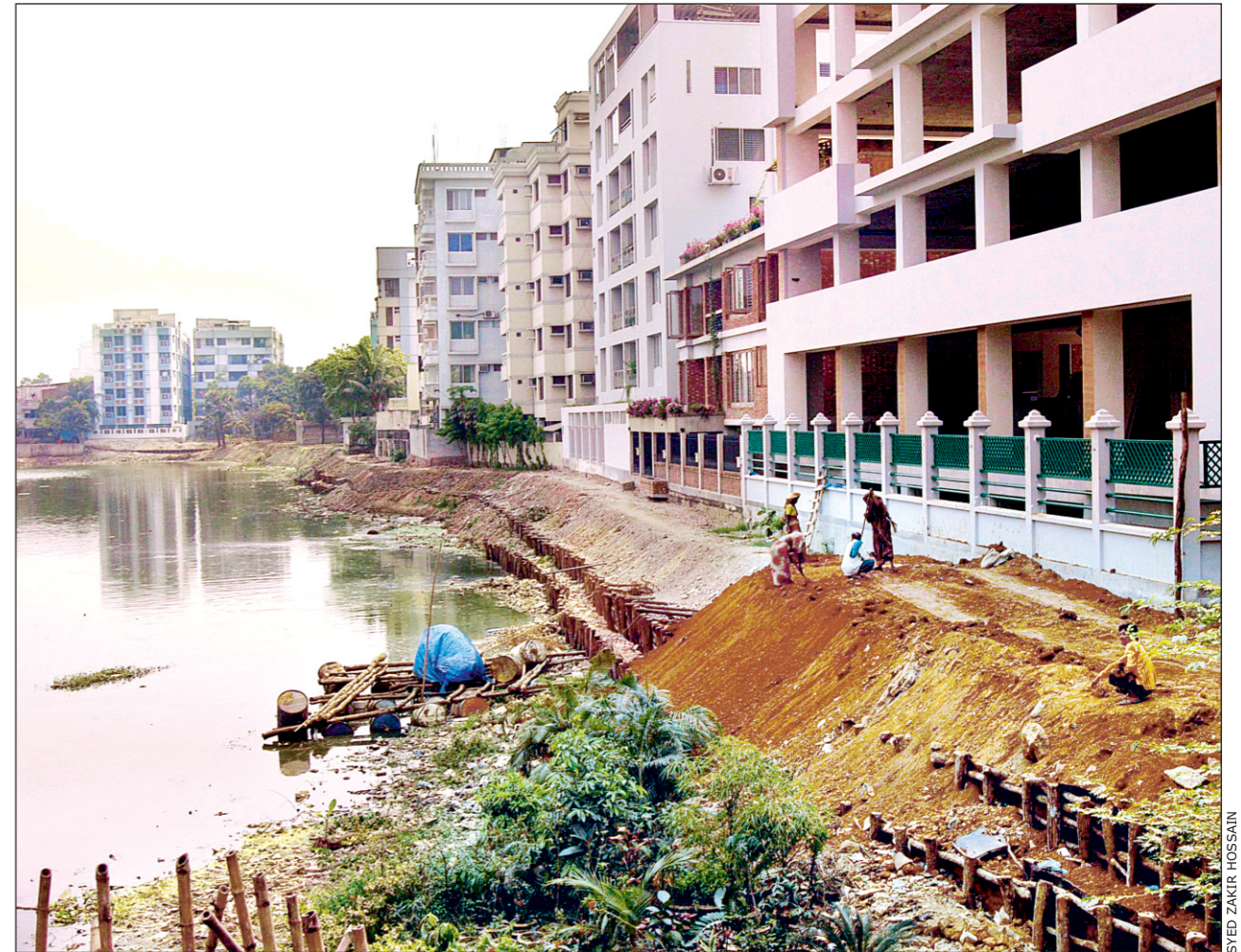
Filling and levelling work to build a walkway along the strip beside the Guishan lake in Banani has begun. This job, which was long overdue, would help in stalling any possible encroachment in the future.
