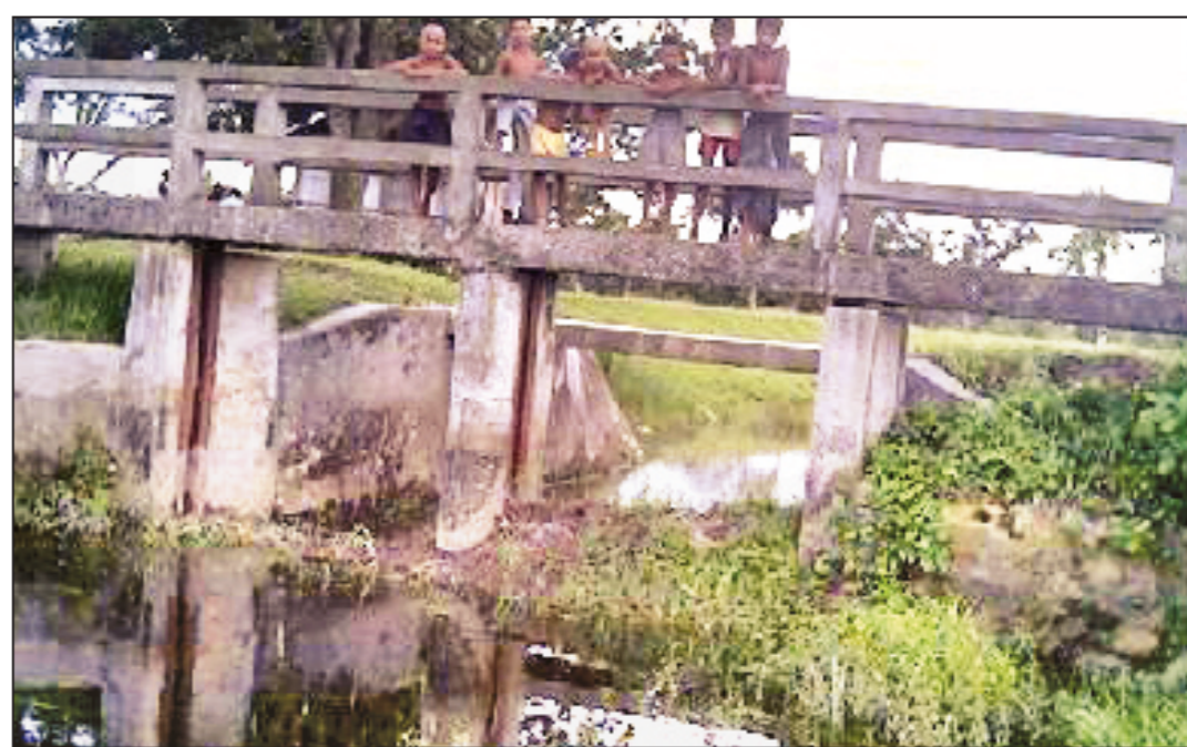
A virtually abandoned sluice gate in Branch Canal-2 of Buri Teesta Irrigation Project at Kaliganj village in Jaldhaka with both its doors stolen.
