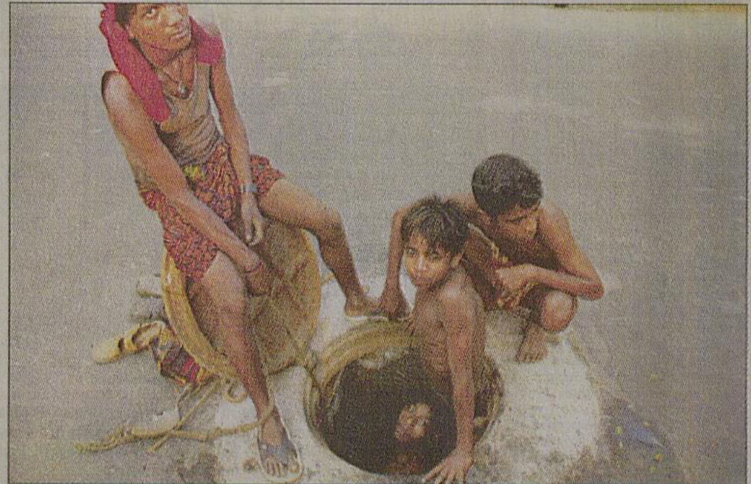
Juvenile workers without any protective gears enter a sewer to unclog it near the Bangladesh Secretariat yesterday. They get Tk 150 each a day for the hazardous work.
