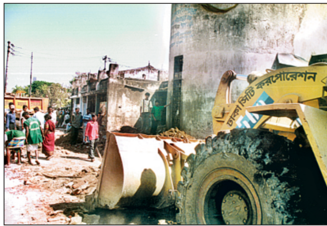
Dhaka City Corporation demolishes several illegal structures of hotels and restaurants at Gulistan in the city yesterday.
