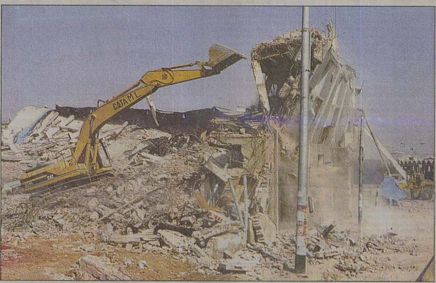
An excavator knocks down a standing part of the collapsed building in Tejgaon in the city yesterday to cut the risk of further fatalities. The disaster on Saturday left at least 18 people dead.
