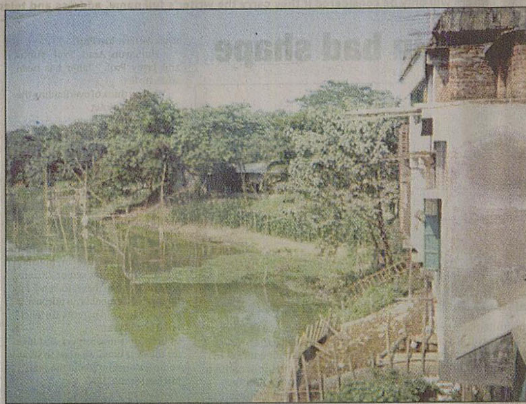
A building being constructed by encroaching the Bairan river in Gopalpur in Tangail.
