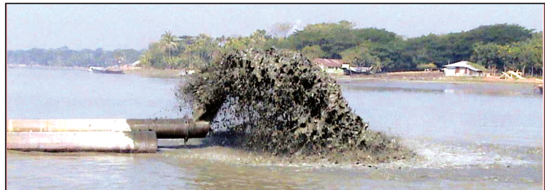
A BIWTA dredger depositing the lifted silt only about 200 feet away from the dredging spot in Patuakhali river.
