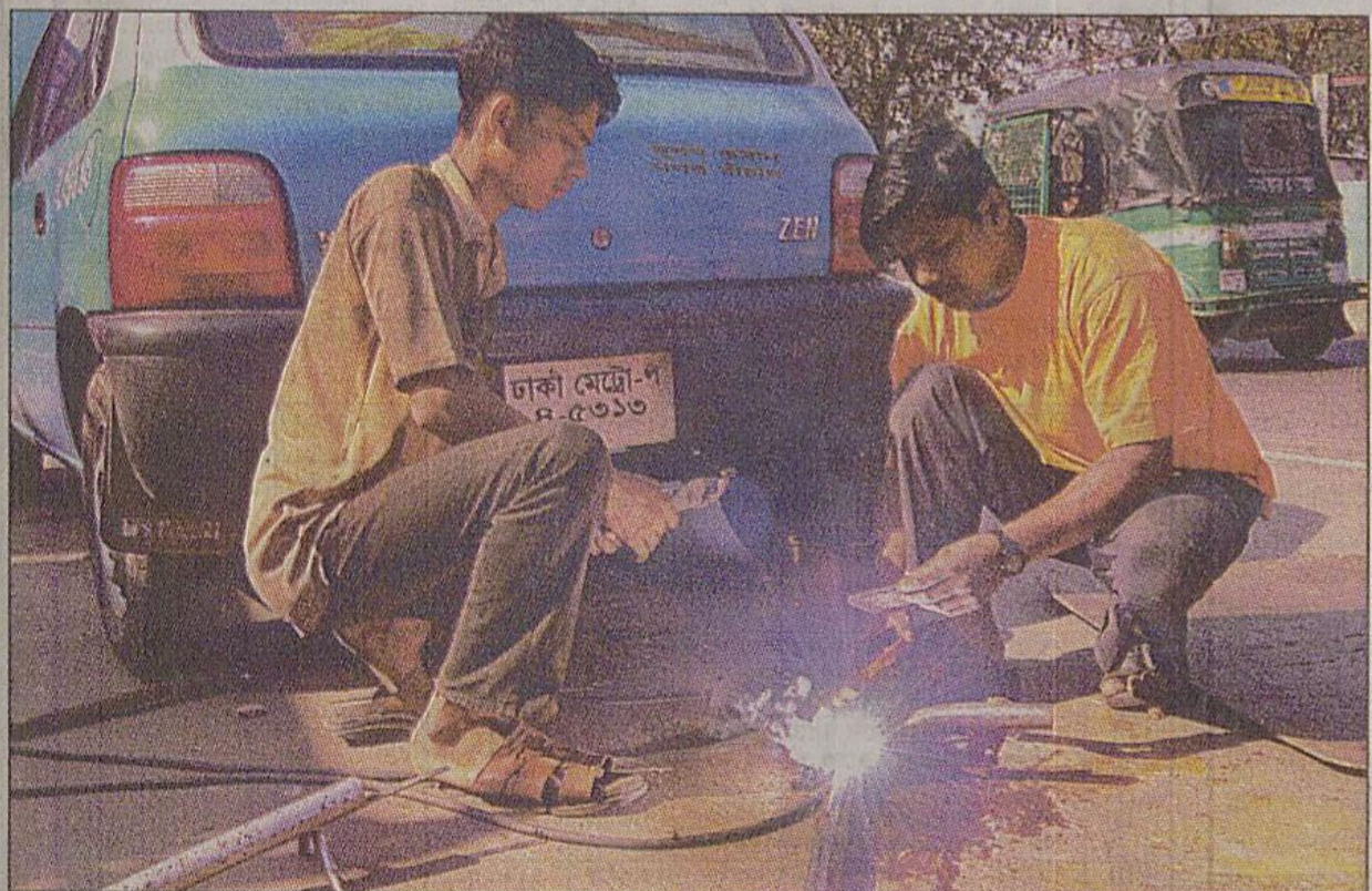
Welding work going on in the open at a workshop in Gulshan.
