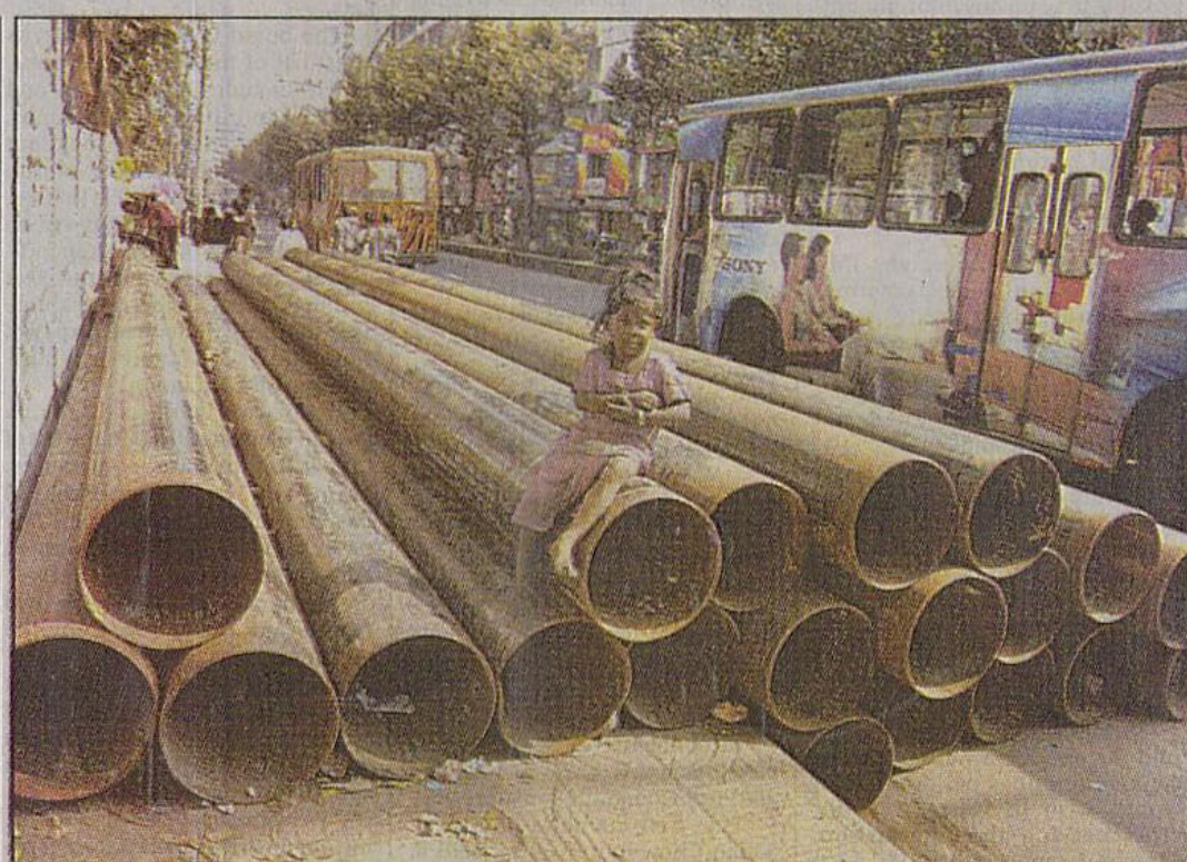
Pipes for underground gas line kept on the road near Science Laboratory for the last one week block the footpath and part of the road.
