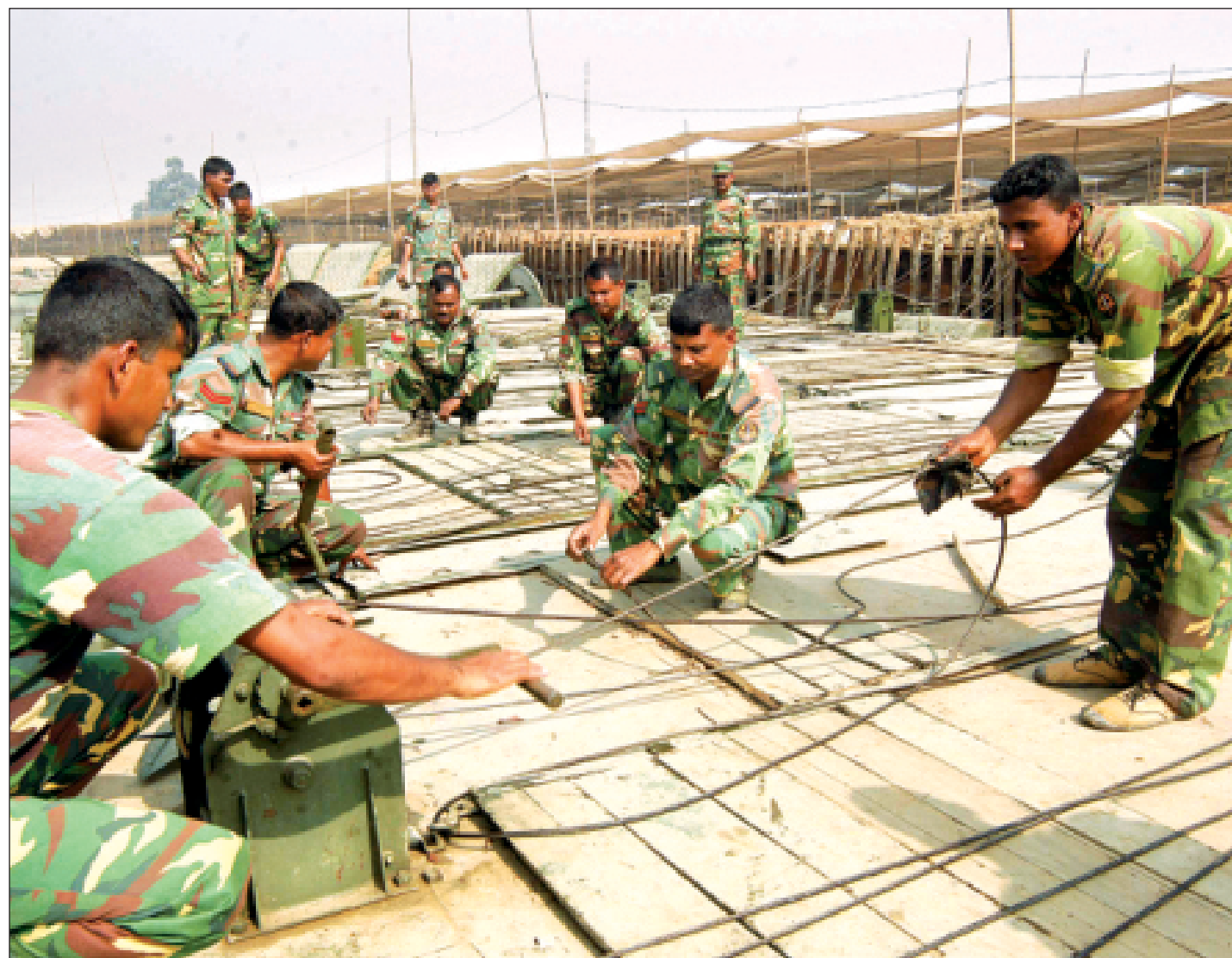
Army men install Bailey bridges on the Turag yesterday so that devotees can cross the river during the three-day Biswa Ijtema, scheduled to start on January 27 in Tongi. PHOTO: STAR
