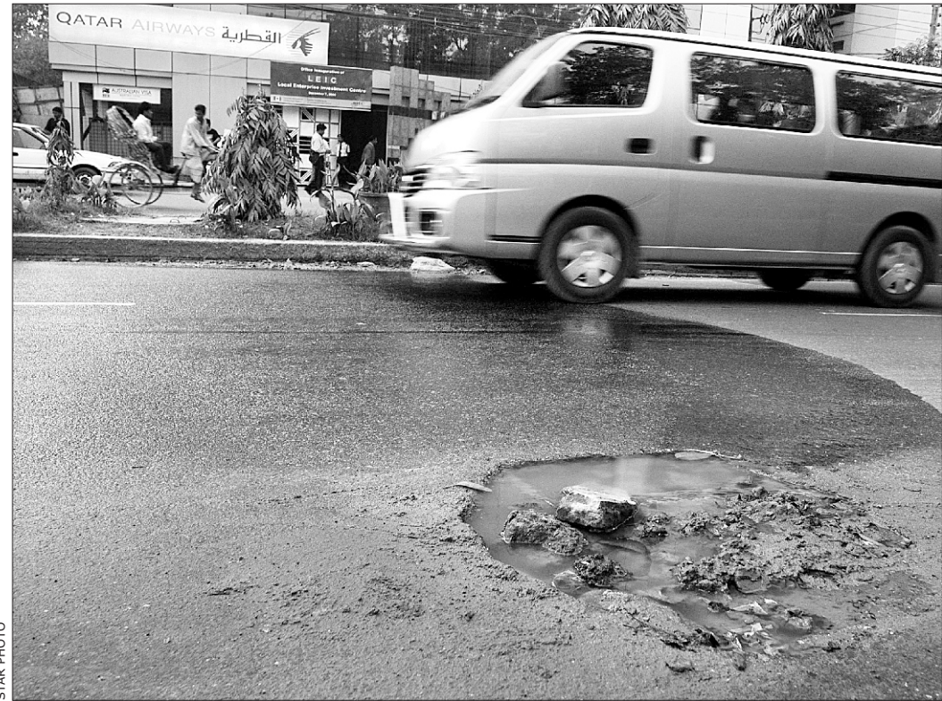
Leaking sewerage in front of Arysha Restaurant in Gulshan 1.
