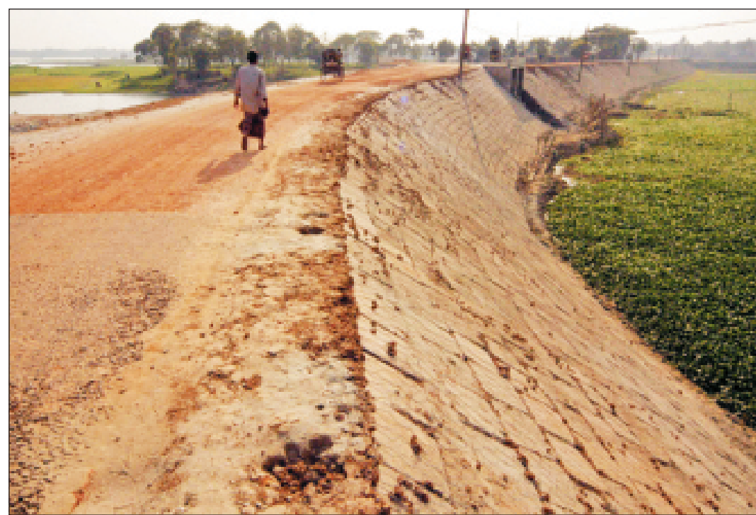
The 1.76 km Mohammadpur-Basila road that is too high and steep for safe journey by pedestrians or vehicles.
