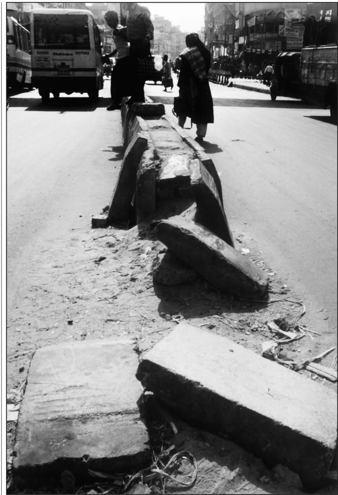
PHOTO: STAR The recently built road divider in front of Fulbaria Railway Station is already falling apart from poor-quality construction.
