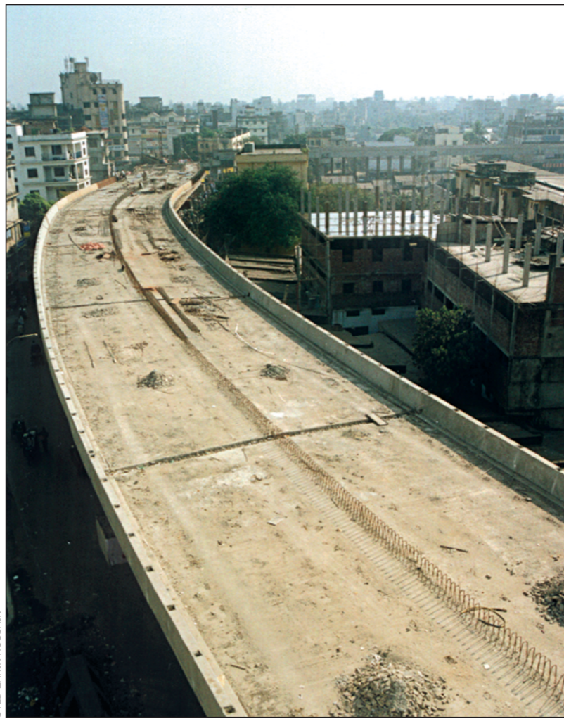
Although part of the under-construction Khilgaon flyover looks almost complete, it may miss the deadline.
