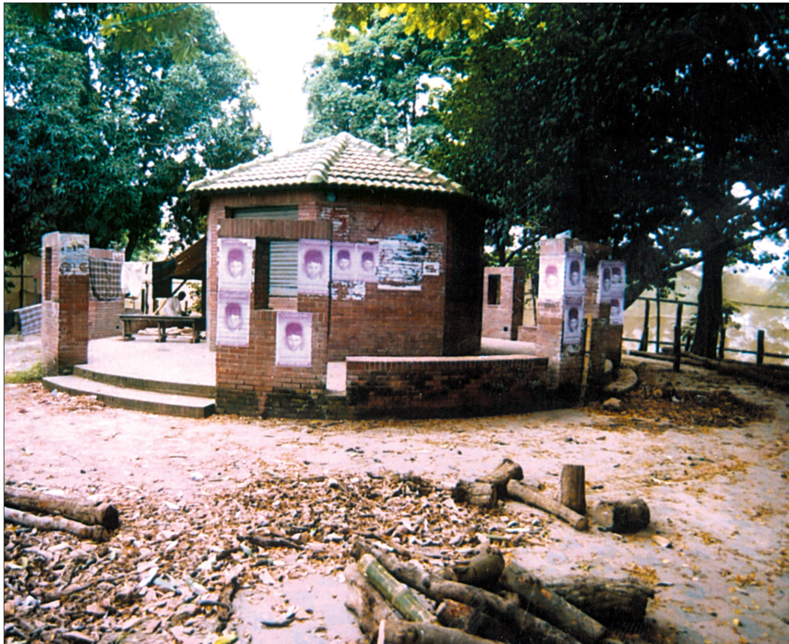
Unplanned renovation is allegedly going on at the food and drink kiosk at Dhanmondi Lake.
