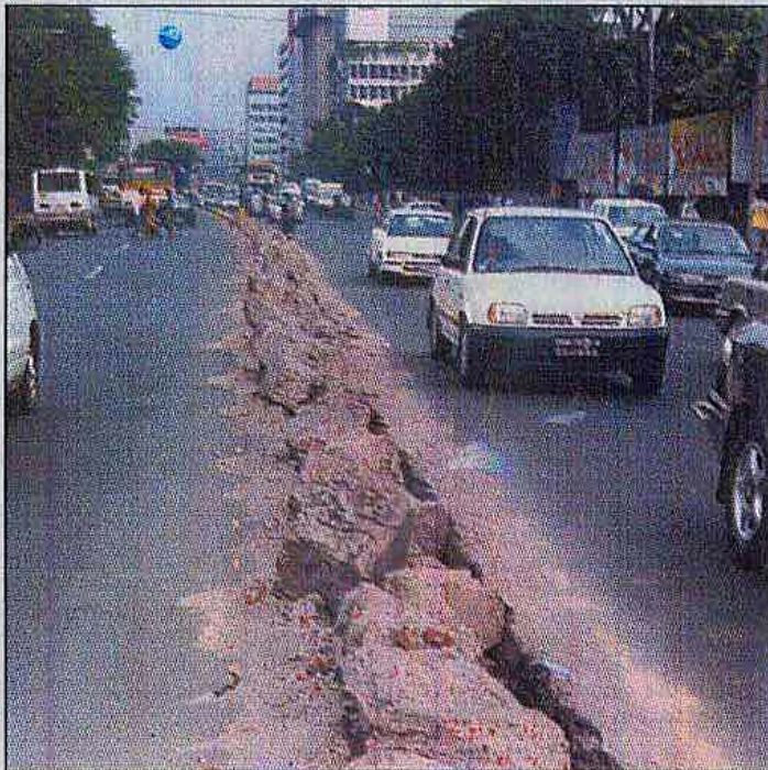
DEJA VU: Fully functional road dividers lie uprooted on Kazi Nazrul Islam Avenue yesterday after authorities tore them down to make room for a new version as part of the road beautification agenda in a waste of state fund.
