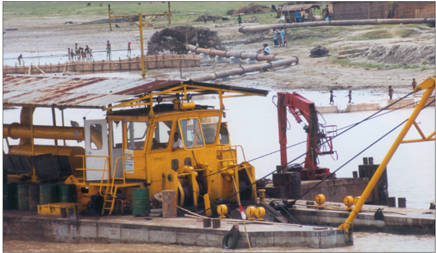
A dredger works at the Paturia-Daulatdia ferry ghat to relieve the Padma river of silt and shoals to open a new channel yesterday. A slide in the water level has forced ferries to carry half the regular passengers and cargo, resulting in long lines of traffic waiting to cross the river.
