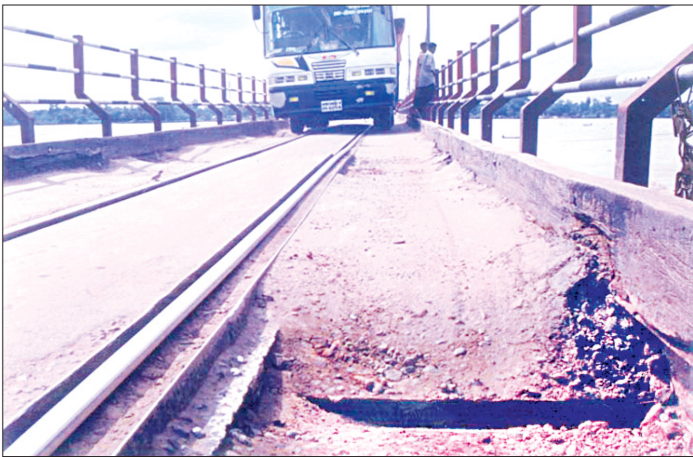
A number of potholes have developed on the east end of Kalurghat Bridge at Boalkhali, worsening its dilapidated state further. Commuting over the century-old rail and road bridge on the river Karnaphuli has become risky nowadays.
