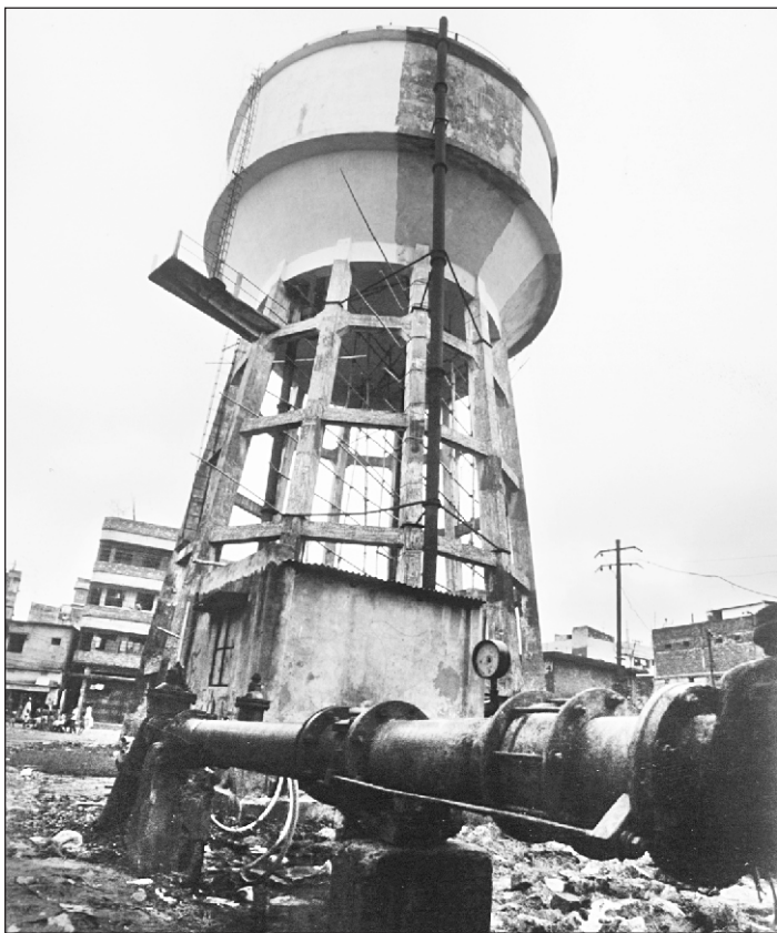
Hazaribagh water reservoir has allegedly not been cleaned for years.
